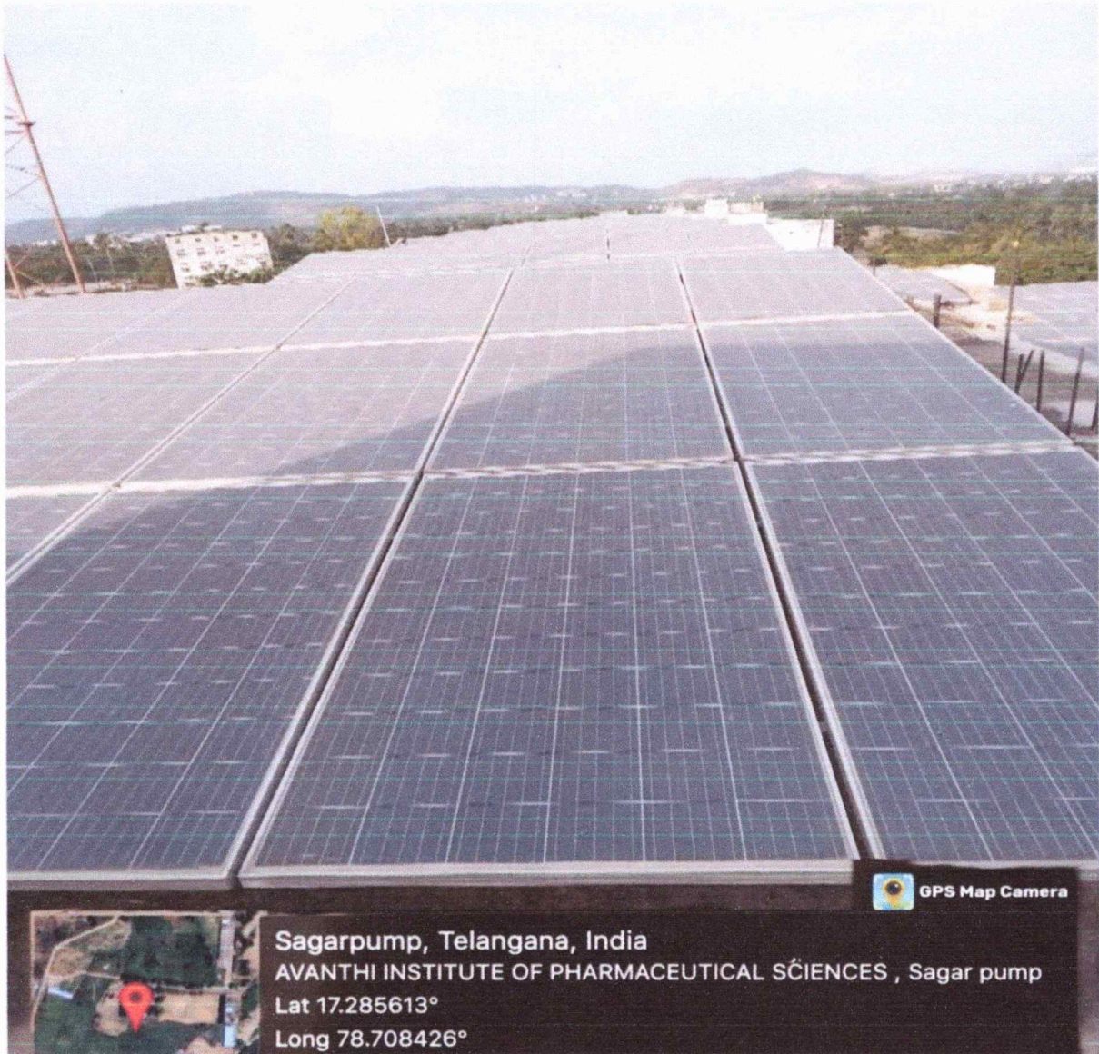
Installed solar panels on top of the Pharmacy Block-I that consist the capacity of 60 KW
