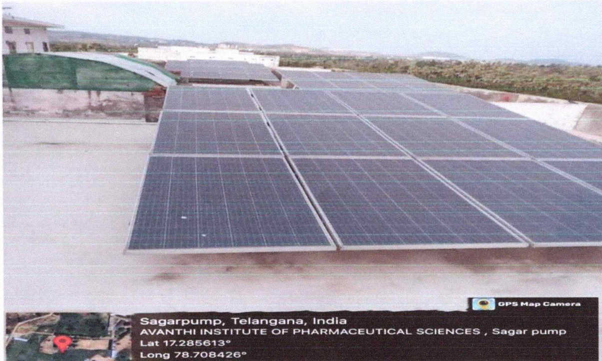
Installed solar panels on top of the Pharmacy Block that consist the capacity of 60 K
