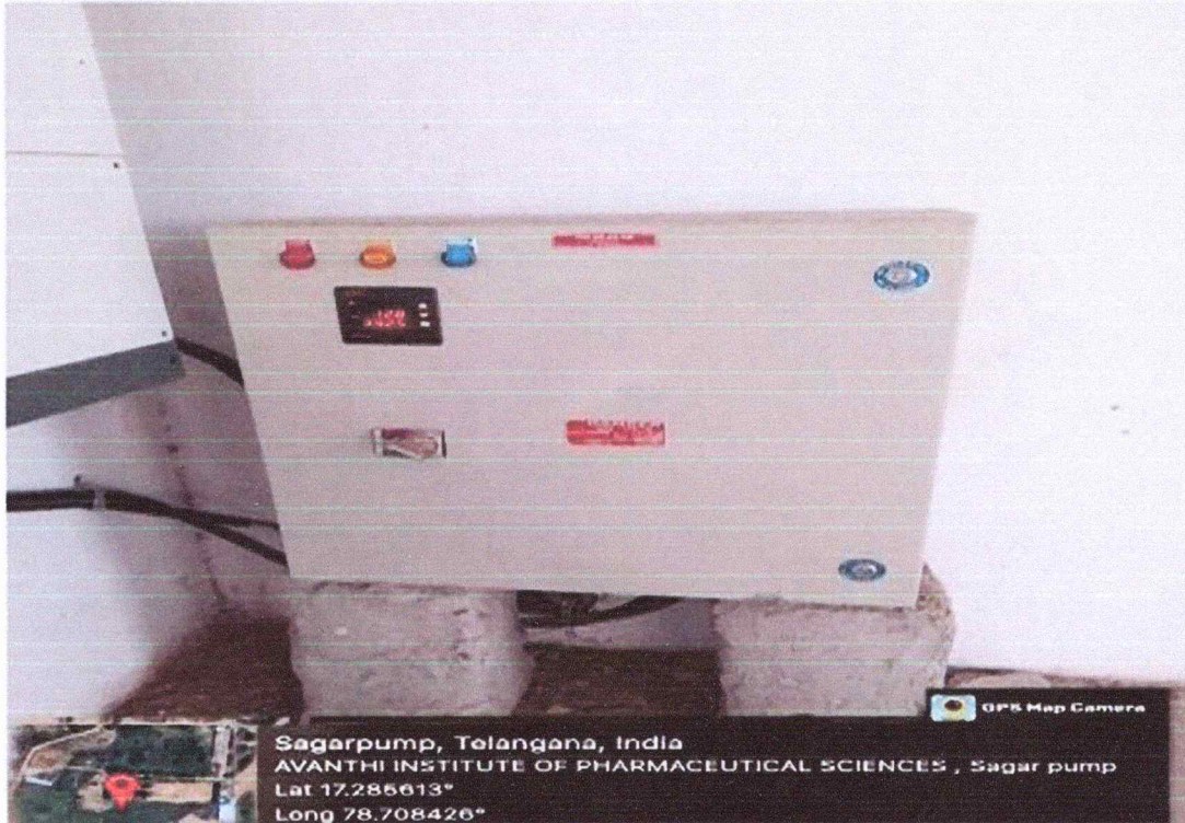
Solar plant connected to power grid
